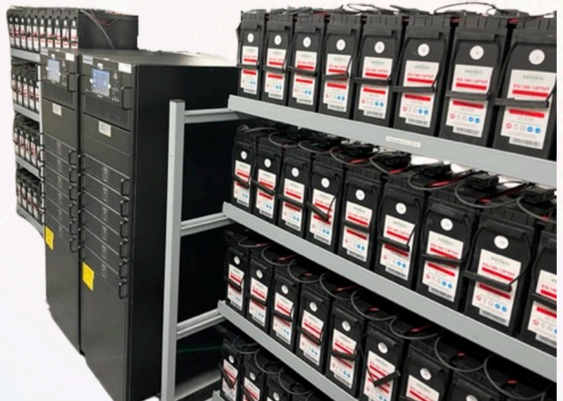
2N parallel Installation
