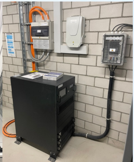
Rack – USV Anlage
